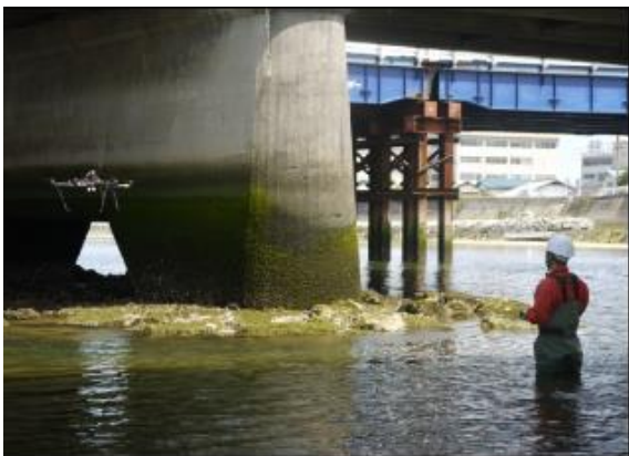
Figure 2. Photographing for an inspection of a lower surface of a bridge girder with manual multi-copter. (a) A crack photo from the multi-copter. (b) The actual situation of operator.
